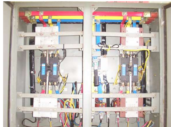
Fig. 5. Remotely operable MCCB Unit at 415 V
