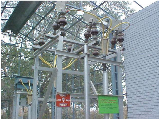
Fig. 4. Load break switch at 11 kV
