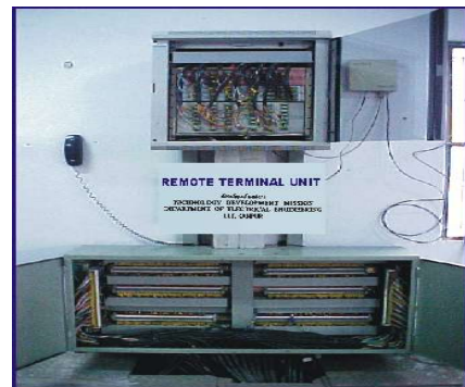
Fig. 3. Remote terminal unit
