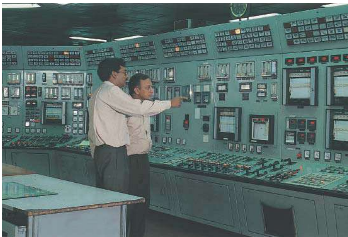
Control room of a power plant
