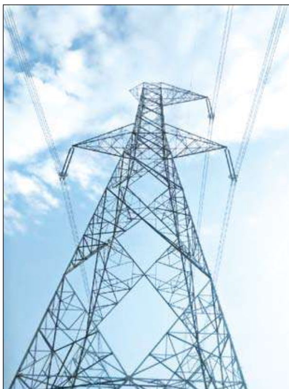
Ghatampur Transmission Line funded by PFC
