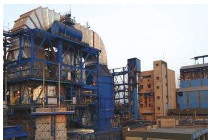
FGD system installed at NTPC Vindhyachal TPS
