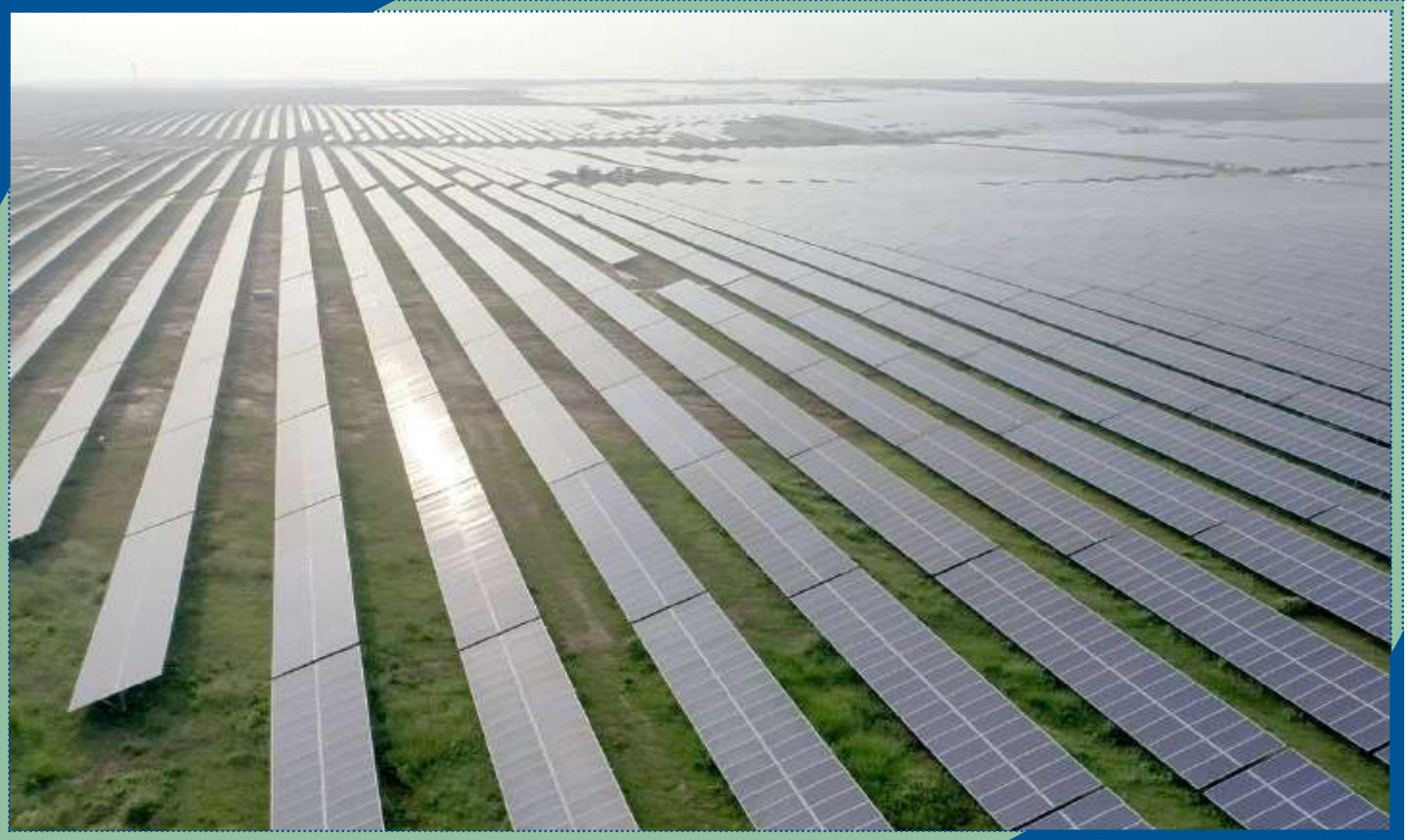
750 MW Rewa Solar Park, Madhya Pradesh
