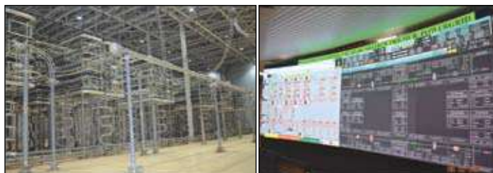
±320kV, 2000 MW, Pugalur – Trichur HVDC Transmission System commissioned in 2021
