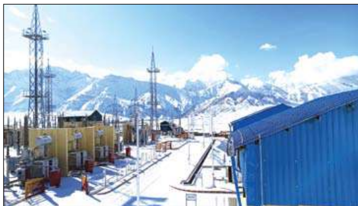
220/66kV Phyang Substation at Leh under Srinagar-Leh Transmission System
