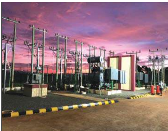
New 2x8 MVA 33/11 KV GIS Substation Mantesh Nagar, HESCOM, Karnataka
