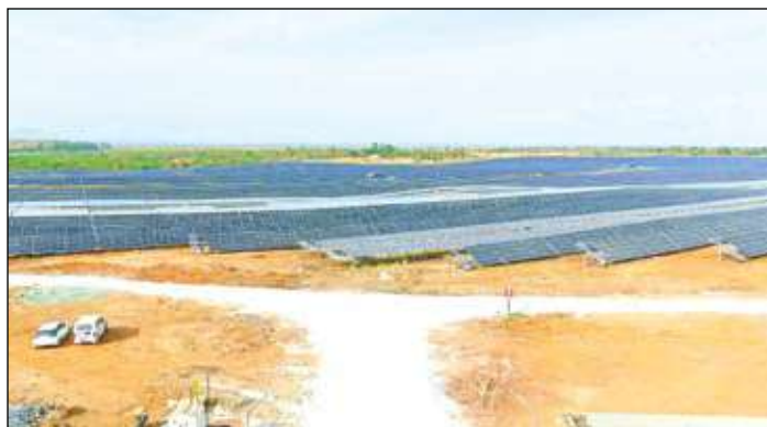
35 MW Babsar Site funded by PFC
