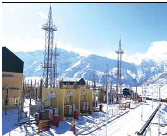
220 kV Phyang, Leh substation
