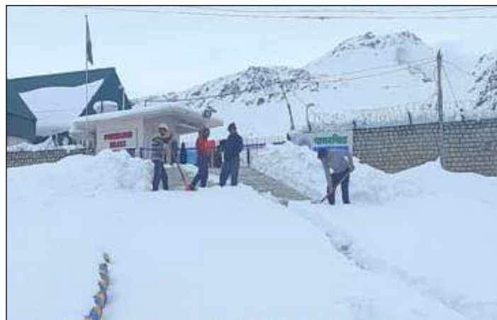
220 kV Drass, Ladakh Substation
