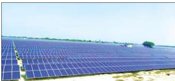
50MW (71MWp) Solar Power Project in Badaun, Uttar Pradesh funded by PFC
